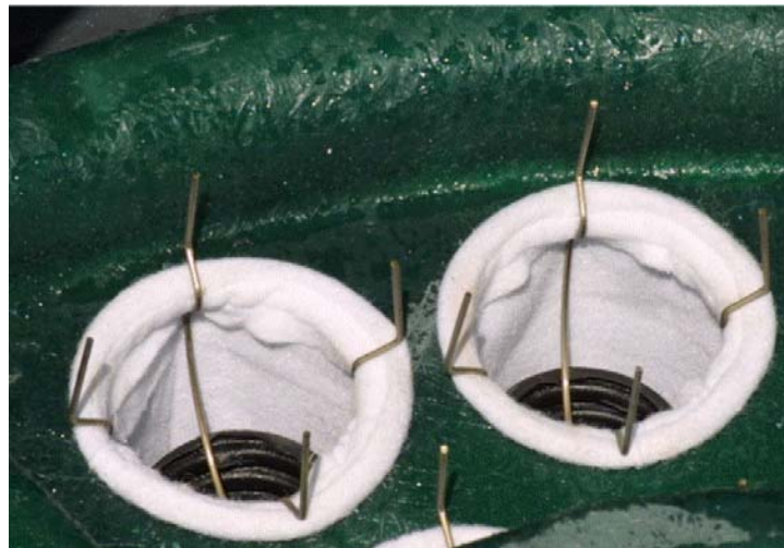
Figure 4—Fixed Film Media and No-Bypass Weir Plate
